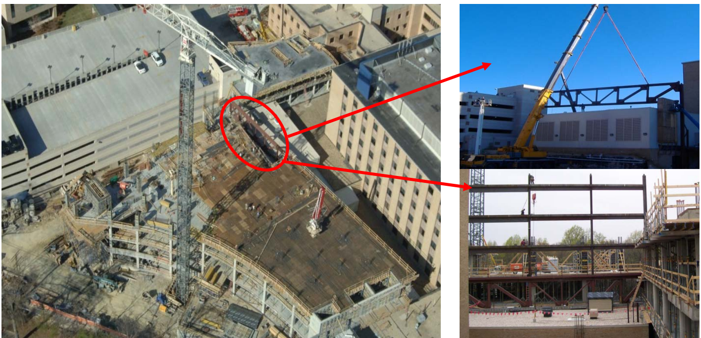
Figure 21: Photos from Patient Tower illustrating the steel truss above the mechanical room
